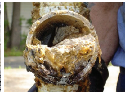
Grease Clog in a Residential Sewer Pipe
