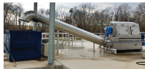
Treatment Plant Bar Screen
