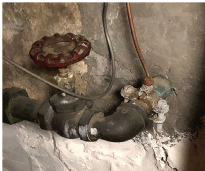
Typical Water Service Line Picture Received from a Customer
